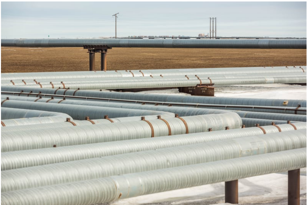
Pipelines at Prudhoe Bay on Alaska's North Slope. (Loren Holmes / ADN archive)
